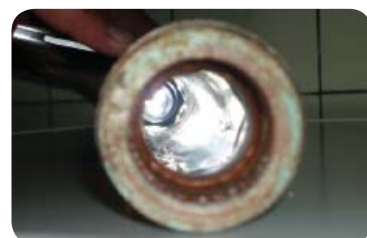
Control hot water pipe after 5 months with Aqua-4D® water treatment
