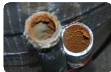
Control pipe in hot water with deposits before installing Aqua-4D®
