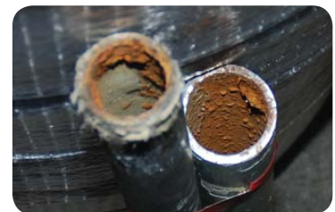
Control tube in the hot water system with heavy deposits before installing Aqua-4D®
