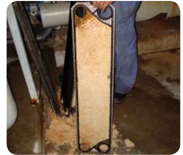
Cost and maintenance problems with limescale in heating circuits
